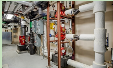
A 58-ton closed loop geothermal system was designed for Fire Headquarters in Branford.
